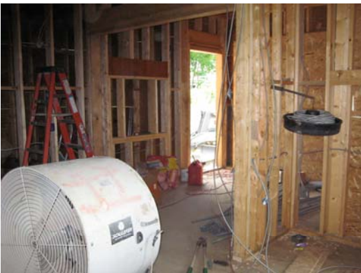
View across part of the lobby. The “inside” box will be where the ATM machine will be. The teller area will be to the left of the ladder.
