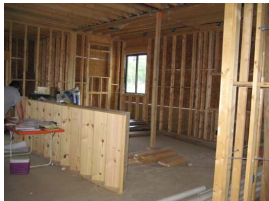
Main teller area. The drive thru window will be to the right of the closely spaced studs (not cut out/installed yet).
